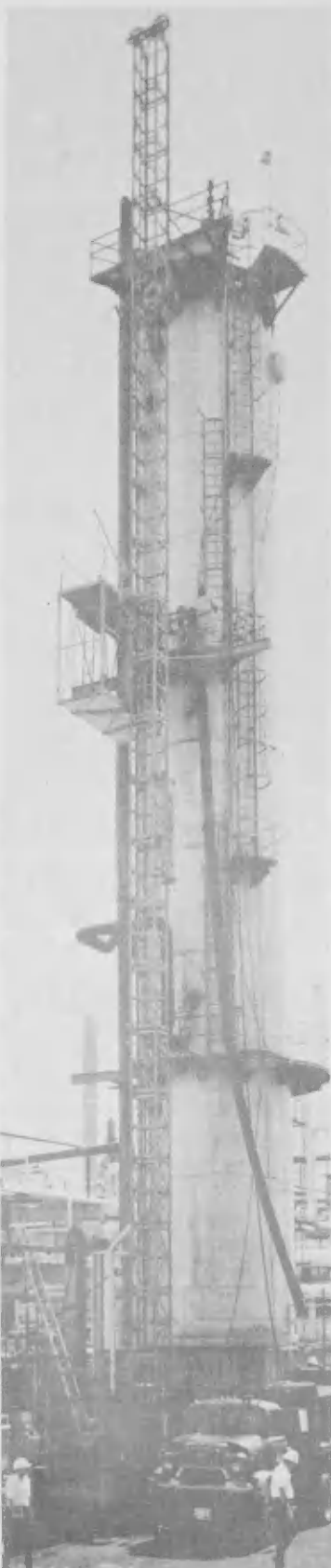
Lago's new Alimak elevator is installed here at the Light Gas Oil Hydrofiner on the HDS site, with its mast extending over the unit's reactor.
